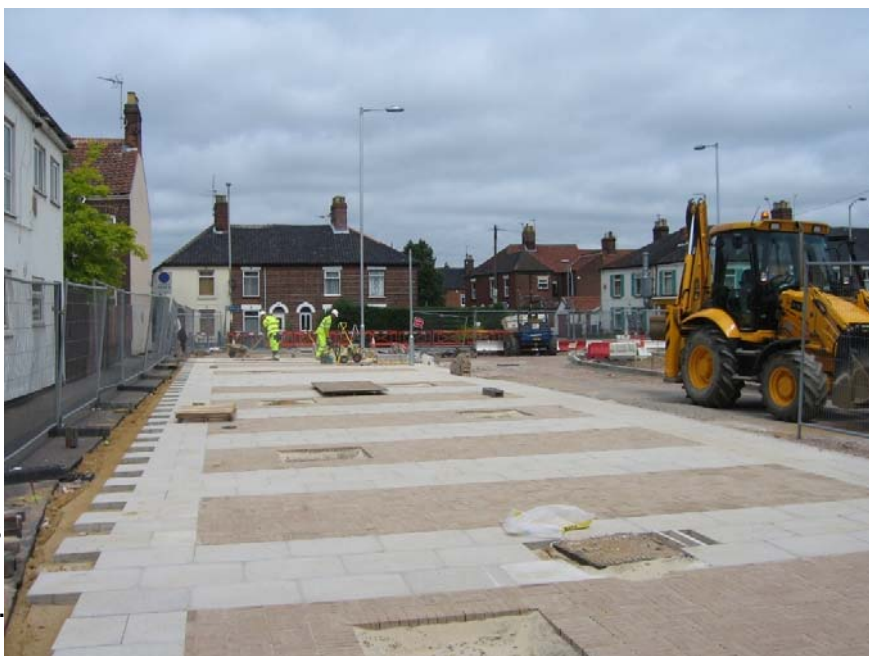
Esdelle Street facing north to Magpie Road showing the new paved area.
